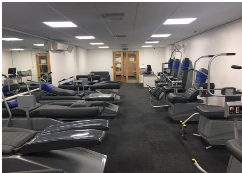
Hatfield Swim Centre - wall removed to integrate a functional training area with the main gym; installed a new functional rig; new Watt bikes; and new flooring, lighting, decoration and wall graphics.
